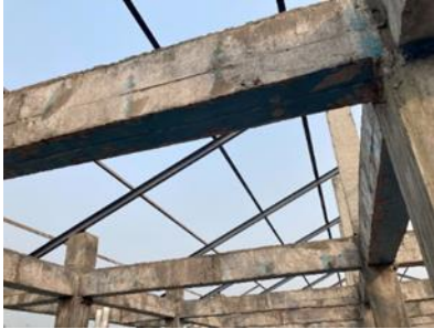
Figure 10: Frame for the pitched roof at the top (Source: Site Survey by Author, 2022)
