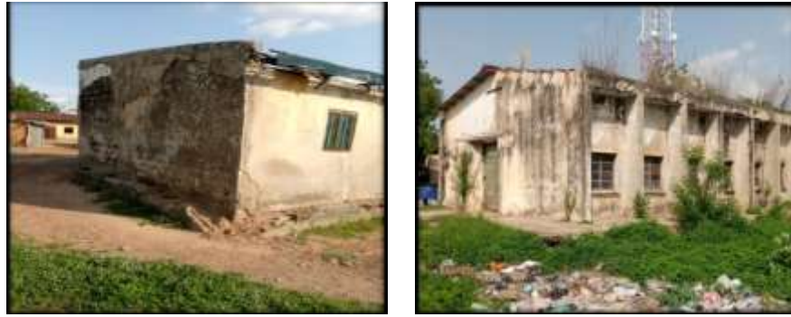
Plate 18: Dilapidated view of the building at Tunga
