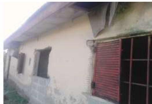
Plate 17: Dilapidated view of the building at Maikunkele pavements at UBEC/NSUBEB Kpankungu
