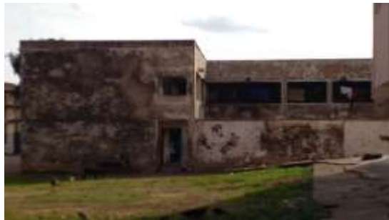
Plate 14: Showing faded walls
