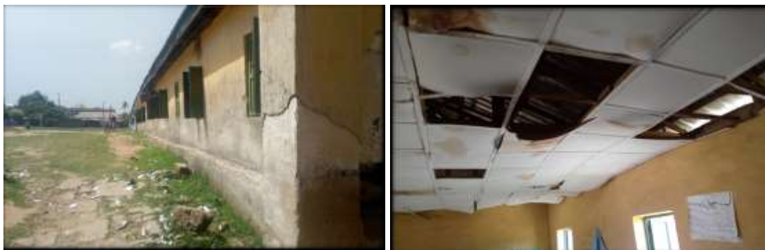
Plate 20: Dilapidating Wall plaster at Bosso
