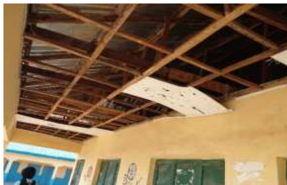
Plate 1: Showing damaged ceilings
