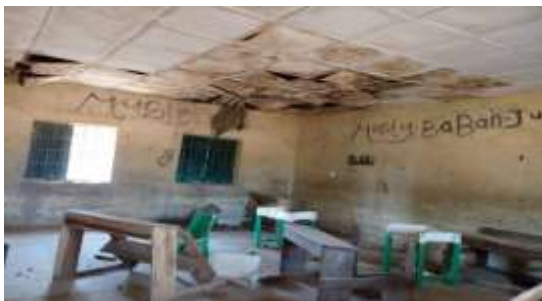
Plate 7: Showing decayed ceiling
